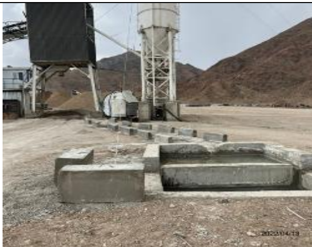
Photo 59. Concrete batching plant's 3-chamber wastewater primary treatment tank at Lot 1.
