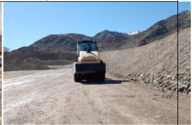
Photo 62 Laying and compaction of clay layer for scarified asphalt disposal site before use.
