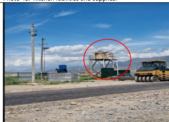
Photo 50. Electrical connections and domestic water supply tanks (inset).
